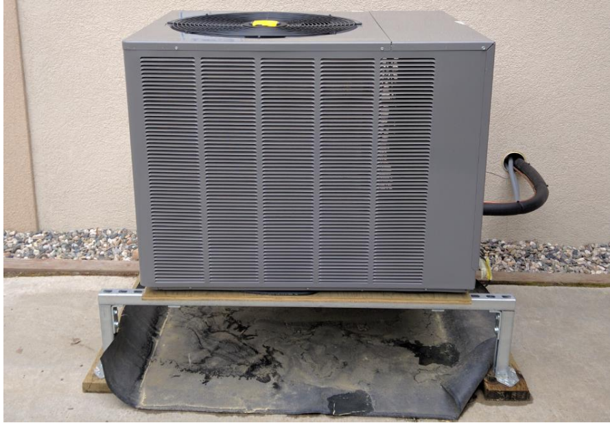
Figure 3: Outdoor Unit of Field Testing Heat Pump in Fairbanks, Alaska
