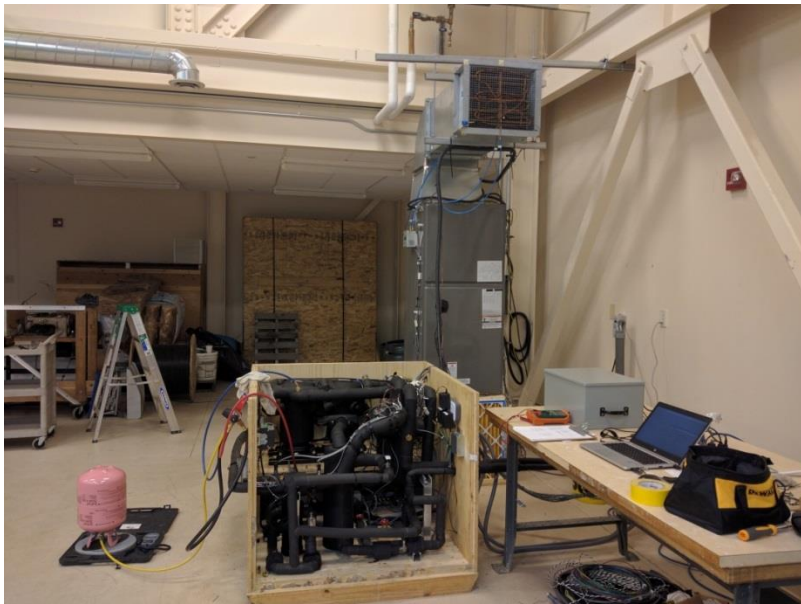
Figure 2: Indoor Unit, Compressor Compartment and Data Acquisition of Field Testing Heat Pump in Fairbanks, Alaska
