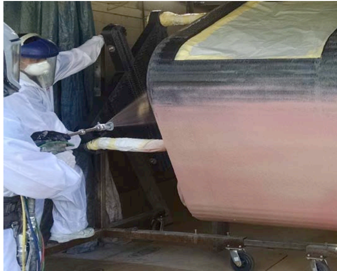
Fig. 6. Spray application of TD Coat RT onto a vertical face of a printed surface.
