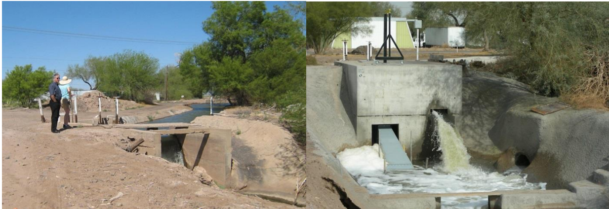
Fig. 4.4. Example of a modular powerhouse for a small, conduit project (concrete box in left photo) installed at a canal drop. (Source: Natel)
