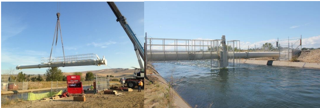
Fig. 6.7. Photographs of the 2013 installation of the spanning beam on the Roza Canal for hydrokinetic testing (left) and the fully deployed, 25 kW Instream Energy hydrokinetic turbine, with the canal running full (right). In this deployment, the spanning beam is structurally independent of the canal. (Source: Instream Energy Systems)
