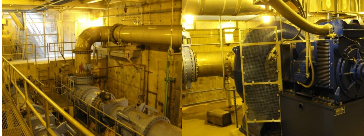
Fig. 6.4. Photographs of the Loring Road project. Shows the original water pipeline on the lower portion of the left side, and new penstock running up and over to new Francis turbine on right. (Source: M.J. Sale, Low Impact Hydropower Institute)
