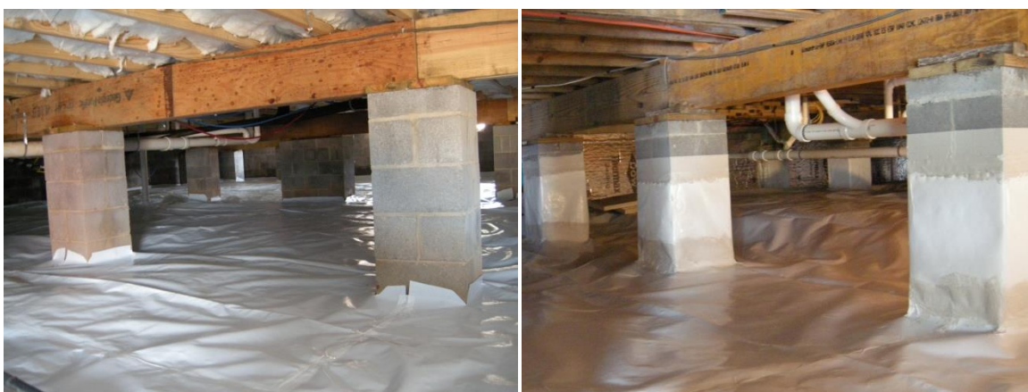
Figure 5. Vented crawlspace in WC3 (left) and walls insulated and sealed in WC4 crawlspace (right)
