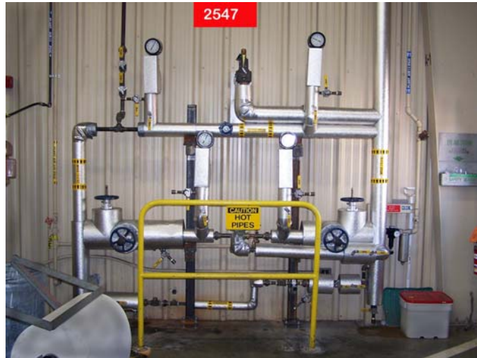
Fig. 1. Newly constructed steam pressure-reducing station.
