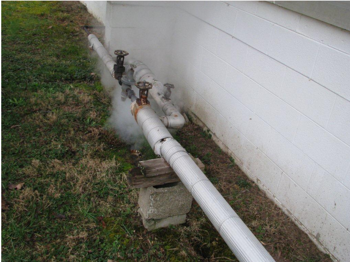
Fig. 2. Leaking steam piping and deficient piping support.
