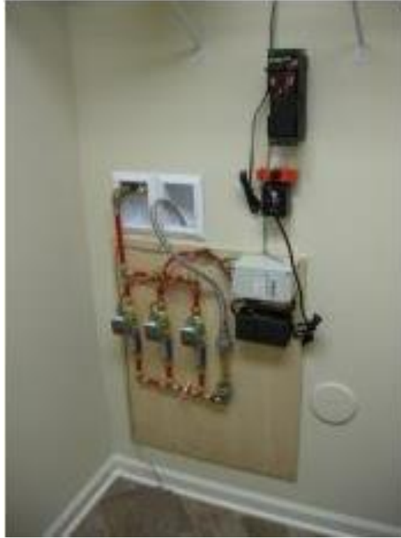
Figure 22. Hot water use control valves.
