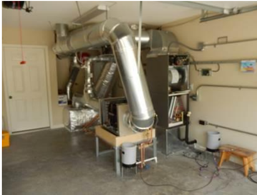
Figure 20. Field-test prototype in installation process. ASHP indoor air handler and WH/DH prototype shown with rain gauges for condensate collection (to monitor DH and latent cooling loads).
