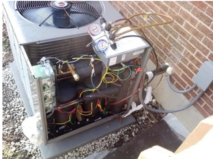
Figure ES-8: Outdoor unit of parallel compressor CCHP field test prototype
