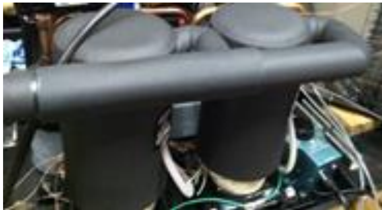
Figure 48: Insulated tandem compressors
