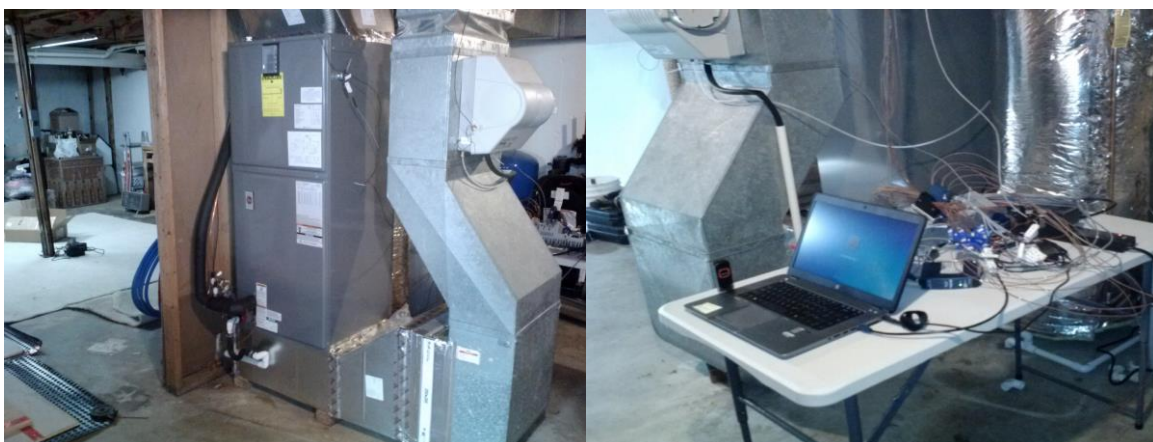
Figure 56: Indoor air handler and data acquisition system
