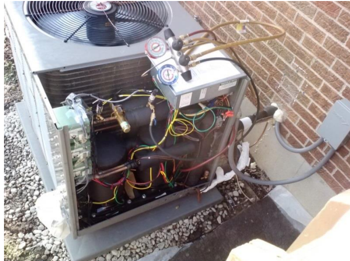
Figure 54: Outdoor unit of field investigation
