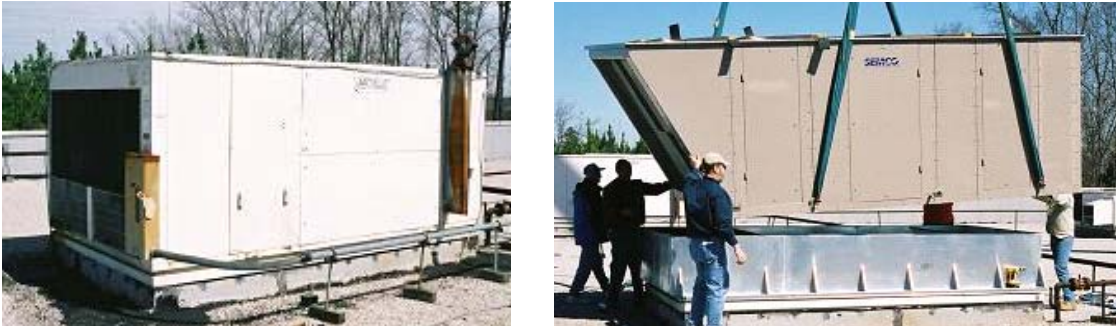
Figure 3. Previous conventional system (left) being replaced by the IADR and curb adapter.
