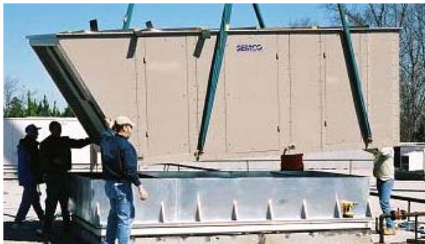
Figure A.1. The IADR system being installed on the footprint used by a conventional rooftop HVAC unit at the Georgia school facility.
