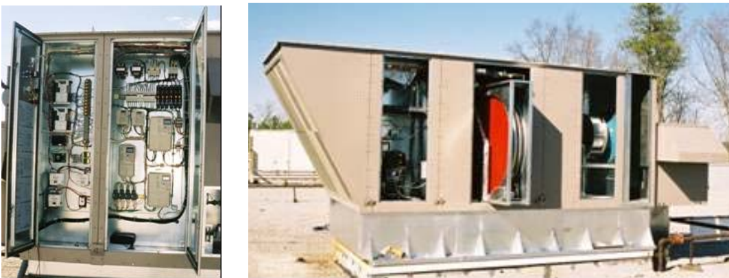
Figure 4. The DDC/data acquisition compartment, desiccant wheel and service access of the IADR unit.
