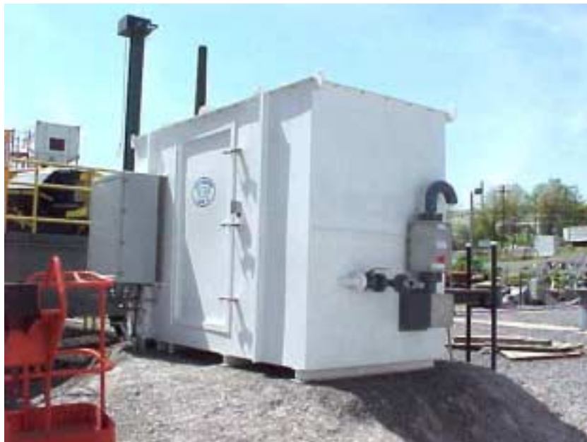
Fig. 4. Primary SCS module.
