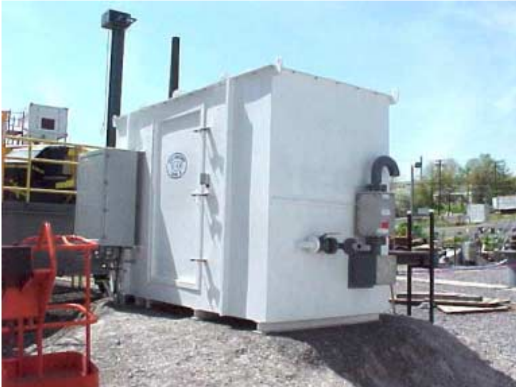
Fig. 5. PCS installed at the GAAT STF.
