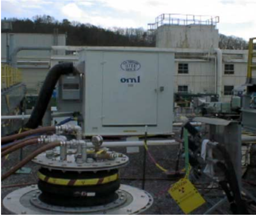
Fig. 3. SMTL installed at GAAT South Tank Farm (STF).
