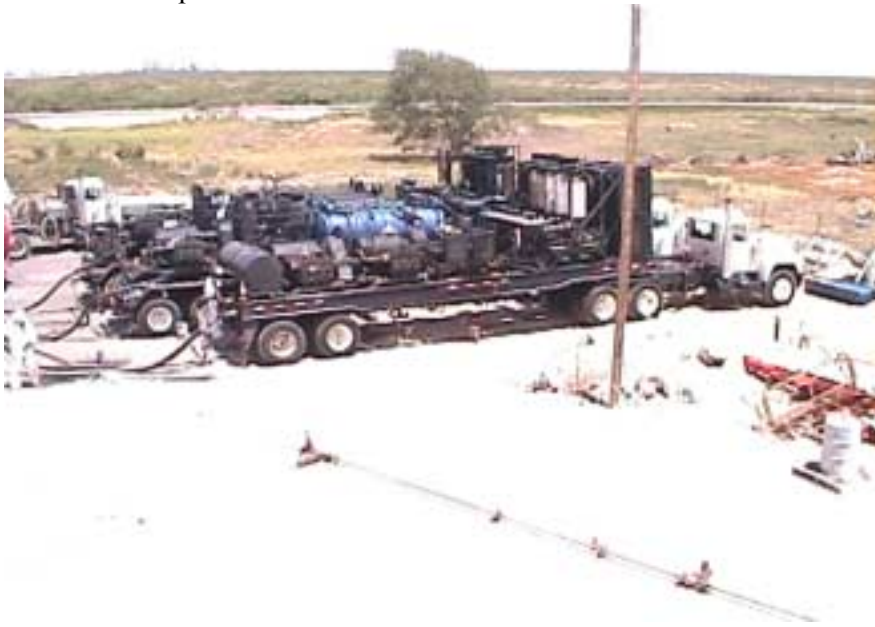
Fig. 9. Overview of equipment used during the FY 1999 MPI cold demonstration in Odessa, Texas.
