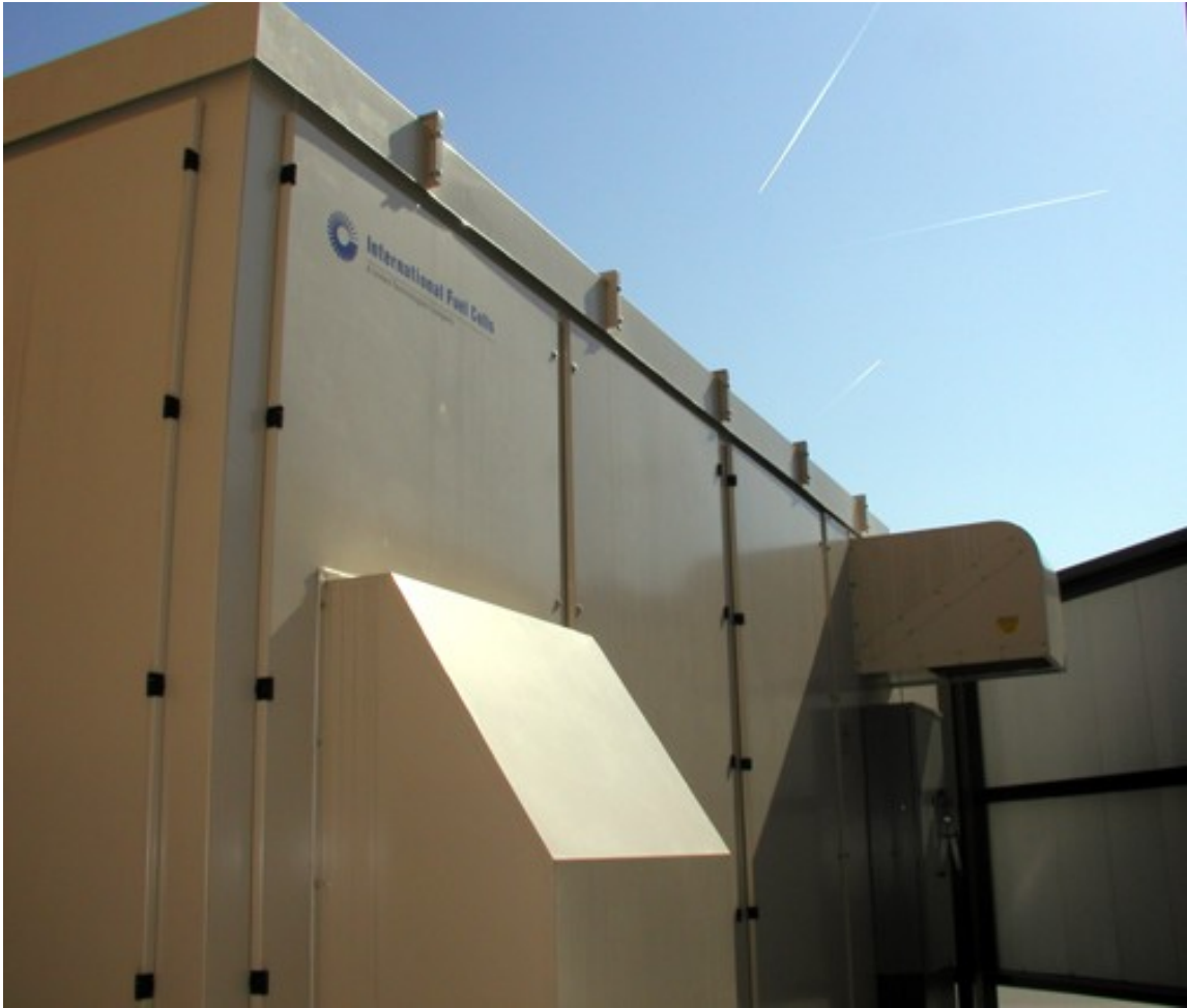
Figure 5. NTRC Fuel Cell Operating
