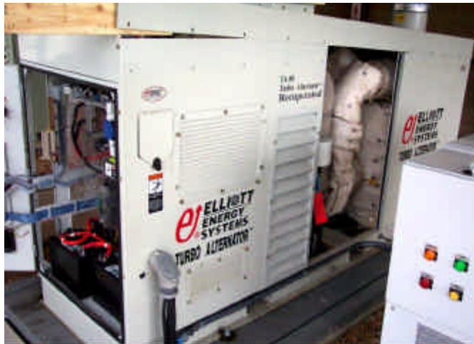
Elliott microturbine (80kW) opened for servicing
