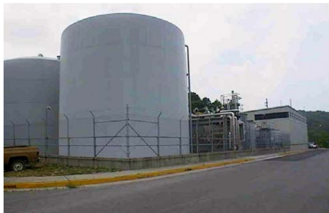
Figure 5-6. Building 3608 and the associated tanks are part of the PWTC located south of White Oak Creek, and are used to treat nonradiological process wastewater.
