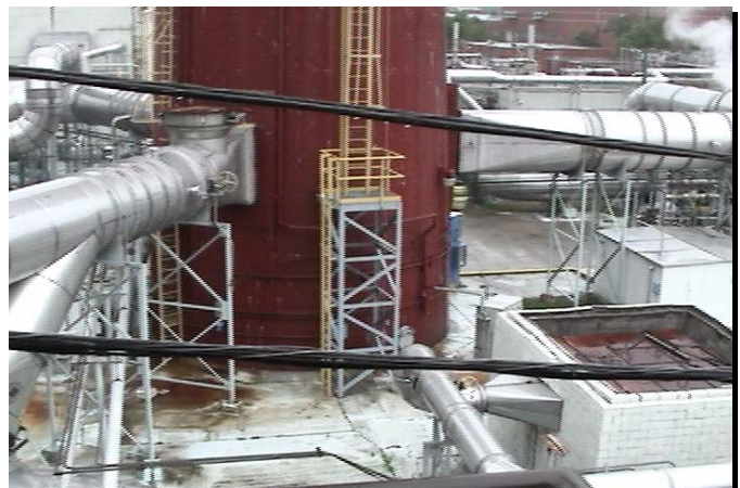
Figure 5-8. Above ground ducts connect into the central gaseous waste system stack, which is located in the ORNL Central Campus.
