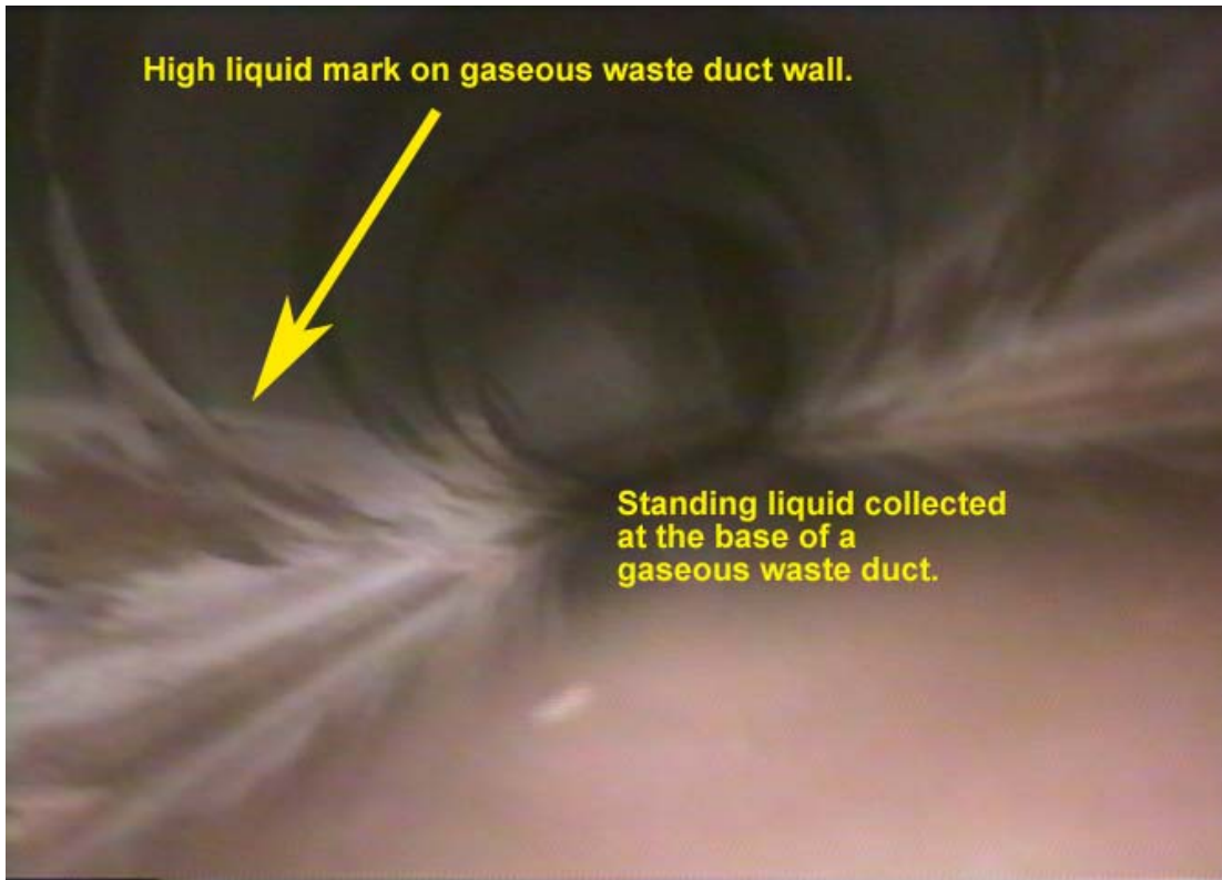
Figure 5-9. Inleakage into the ORNL gaseous waste system ductwork was found during a 1996 video inspection.
