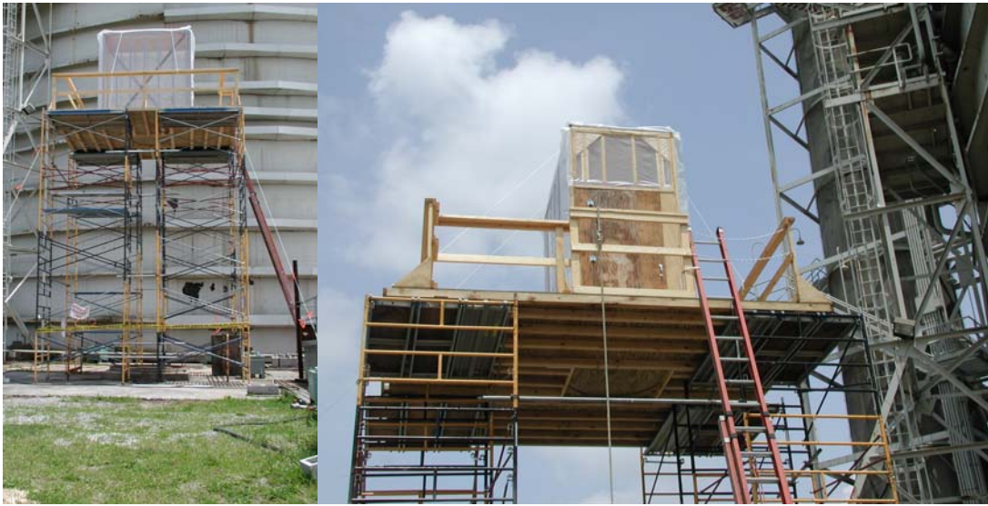
Fig 2. Test platform for long-reach tool at ORNL.
