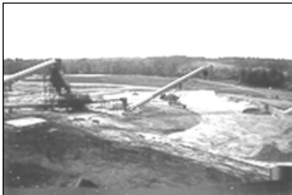
Figure 19. An Example of a Radial Stackers Loader with the Storage Currently Empty.
