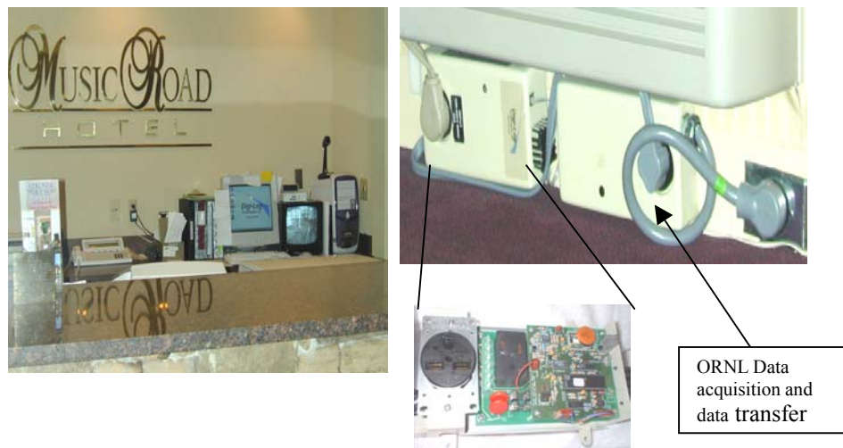
Fig. 5. Clockwise from left: front desk controller at motel, installed Digi-Log unit and control board, ORNL data processing and data transfer module.
