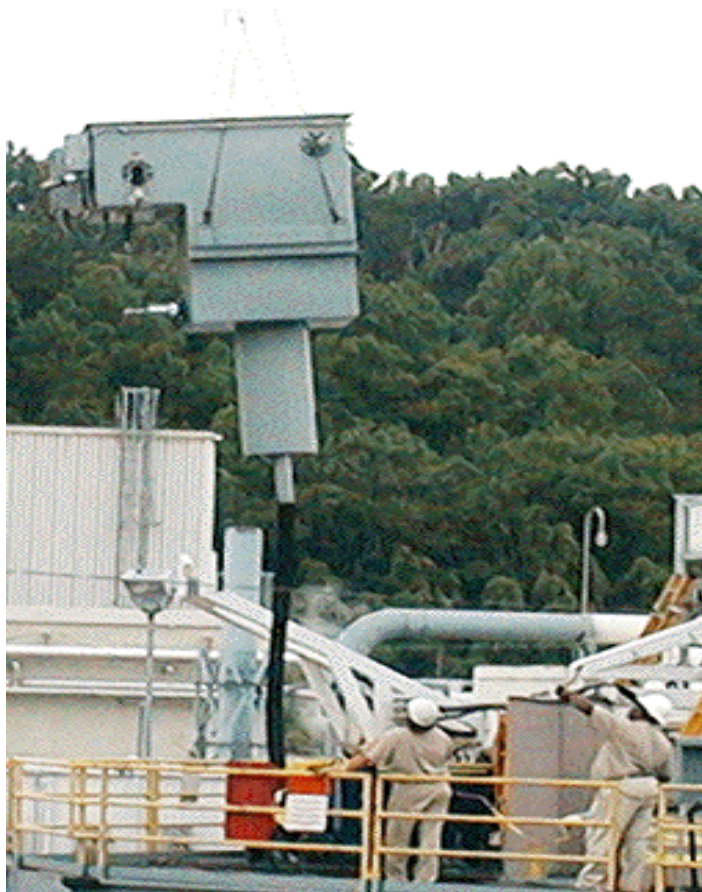
Fig. 6. WaRTS surge tank and confinement box assembly as it is lifted onto a riser of tank W-9.
