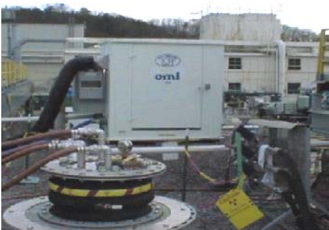
Fig. 5. SMTL enclosure with top of PAM system in foreground at GAAT W-9.
