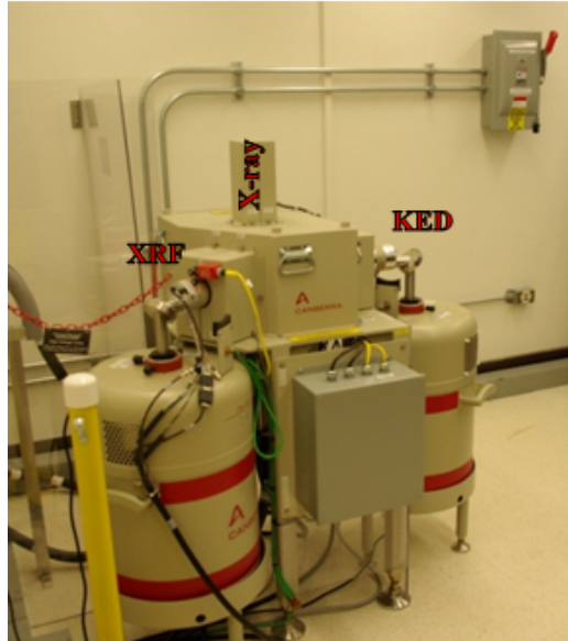
Figure 8. HKED system installed at the Radiological Engineering Development Center facility in ORNL. (Photo courtesy of R. D. McElroy, ORNL.)
