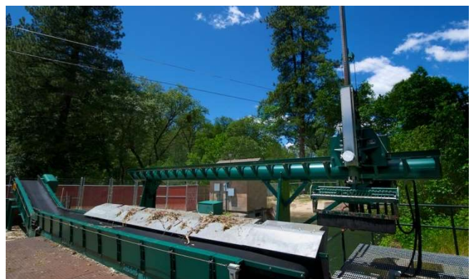
Figure 24. Trash rake conveyer system (courtesy of Atlas Polar Co.).
