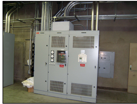
Figure 29. Typical solid-state cabinets.
