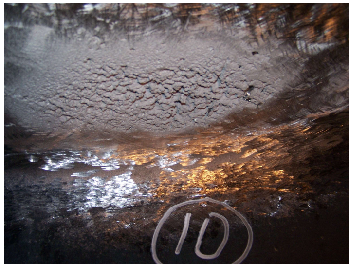
Figure 96. Typical cavitation damage to runner blade.
