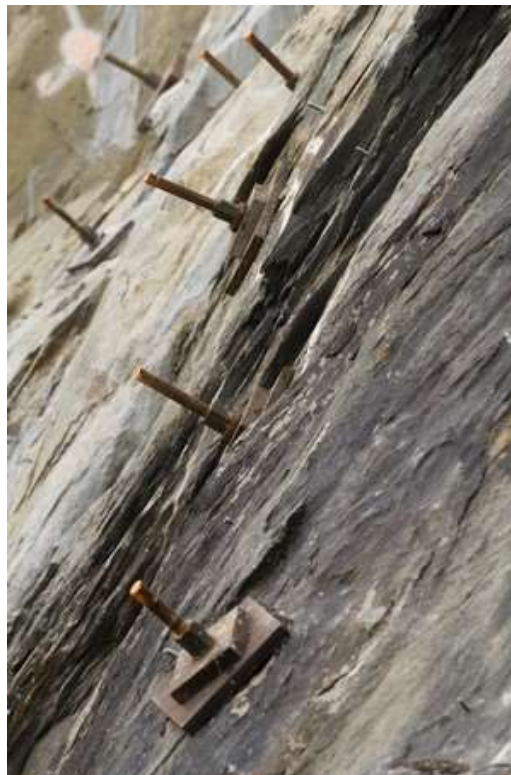
Figure 8. Slope stabilization (Ocoee River Flume, Ocoee, Tennessee). Photo Courtesy of J. Miles Cary.
