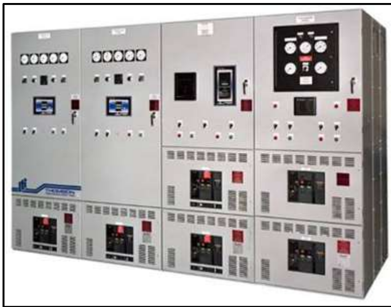
Figure 54. Typical switchgear lineup for station service power system.
