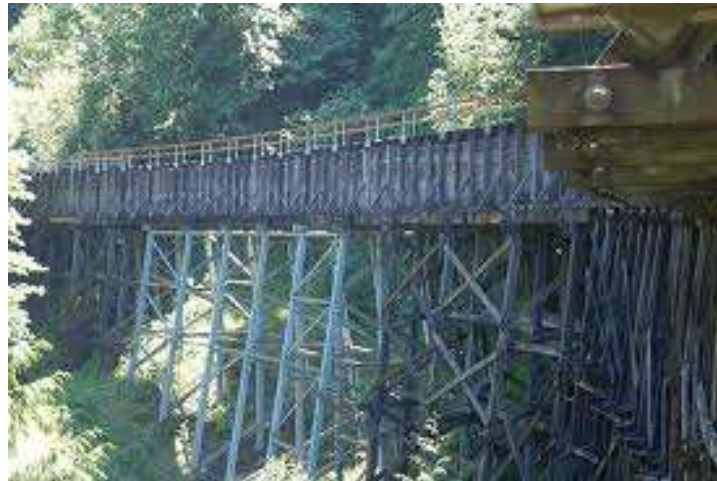
Figure 5. Wood flume (Bull Run Hydro Project, Oregon).
