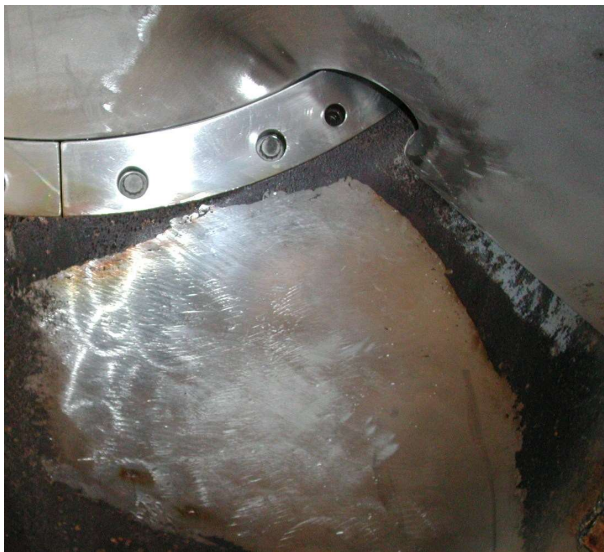
Figure 137. Stress relief notch and overlay.
