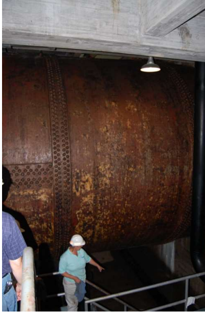
Figure 17. Exposed portion of penstock at Center Hill Hydro Plant (DeKalb County, Tennessee).
