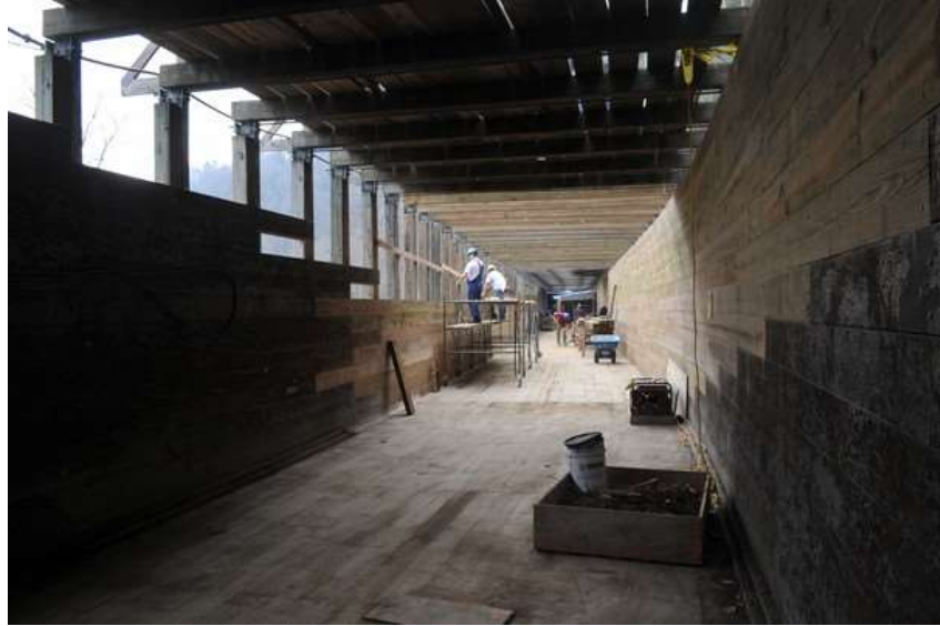
Figure 9. Wood flume repair (Ocoee River Flume, Ocoee, Tennessee). Photo Courtesy of Jason Huffine/TVA.
