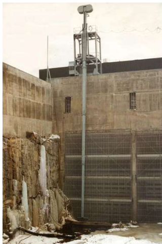
Figure 23. Trash rake system (courtesy of Alpine Machine Co.).
