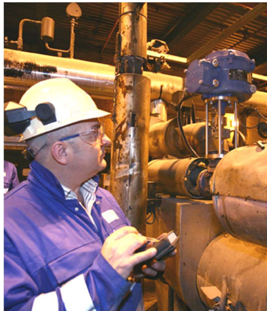
Figure 149. Typical collection of data from the control valve assembly.
