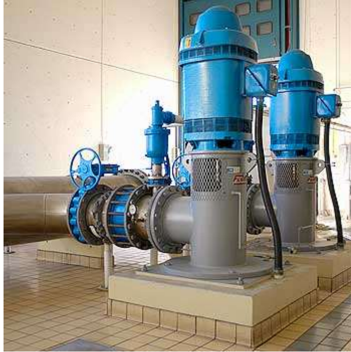
Figure 171. Typical dual raw water pump setup.
