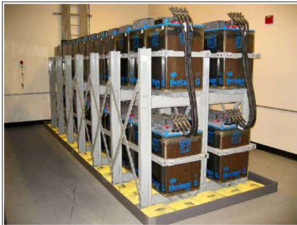
Figure 55. Lead acid batteries in a bank.
