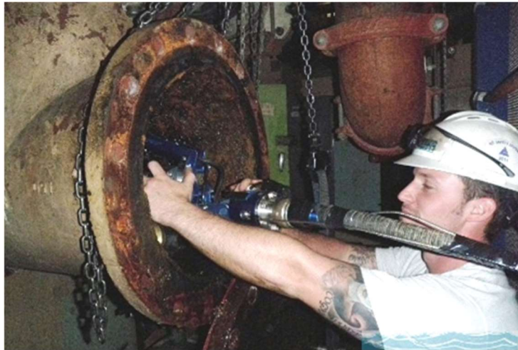
Figure 173. Remote operated vehicle for pipeline inspection of raw water system (Substructure, Inc.).
