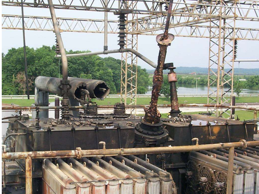
Figure 51. Results of single 500-kV bushing failure.
