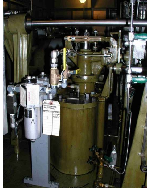
Figure 124. Pilot valve duplex strainer.
