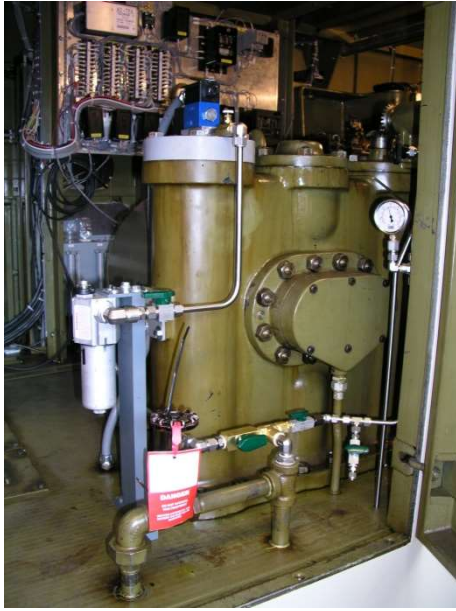
Figure 123. Pump un-loader pilot valve and strainer.
