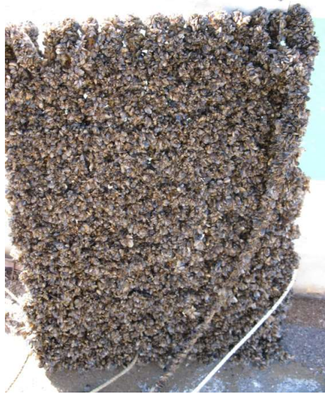
Figure 16. Invasive zebra mussels on steel surface.
