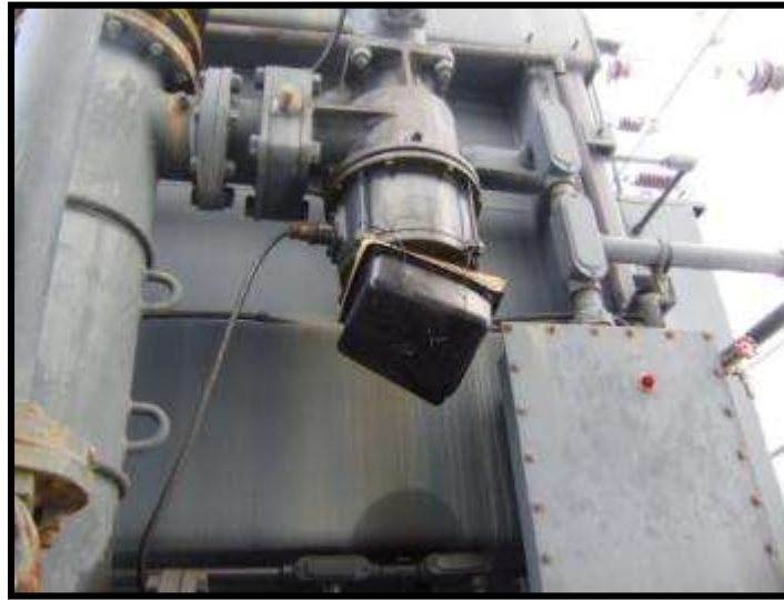
Figure 50. Excessive oil leak on motor-driven oil pump.
