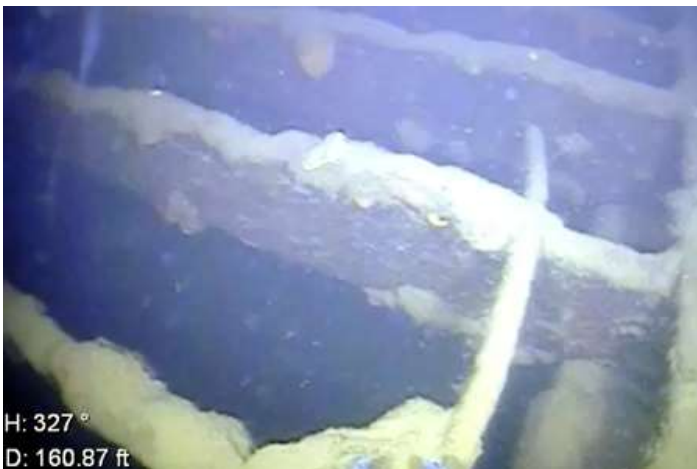
Figure 20. ROV still image of trash rack.*
