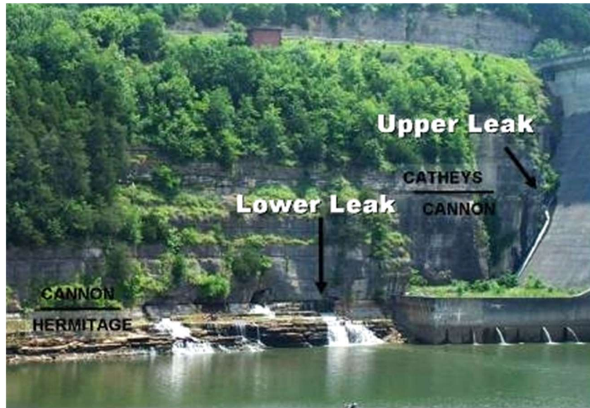
Figure 11. Appearance of leakage (Center Hill Dam, Tennessee) [7].
