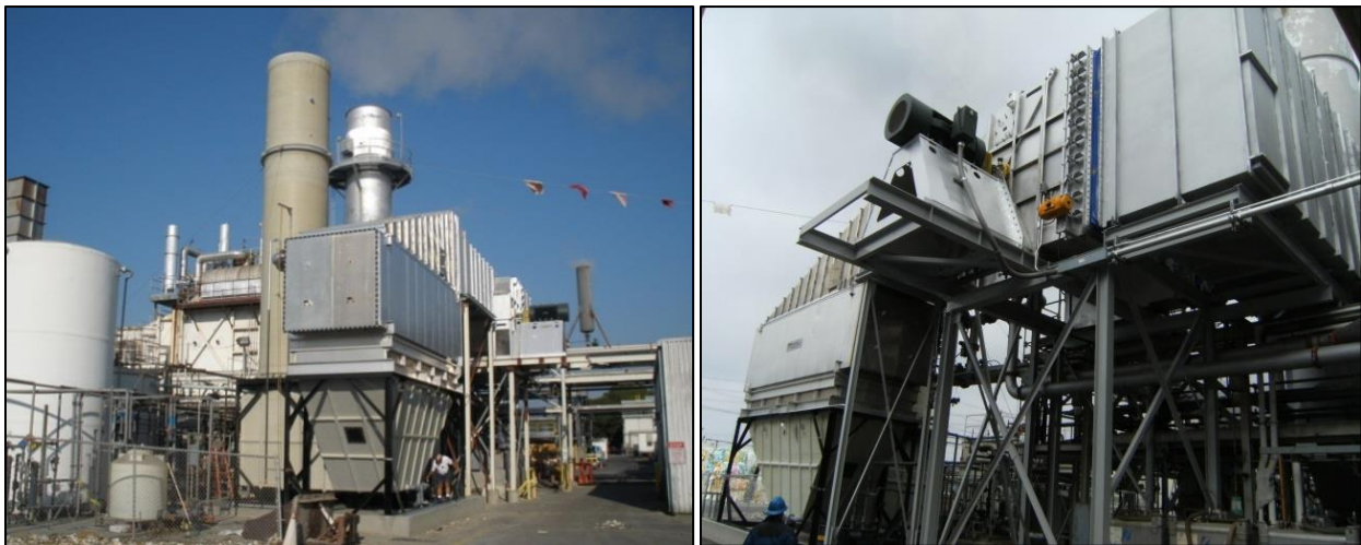
Figure 3-6: Installation of a noncontact condensing economizer at a chemical plant. Courtesy: Combustion and Energy Systems, Ltd.
