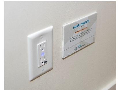
Altus Home Smart Receptacles. Image courtesy: Georgia Power .
