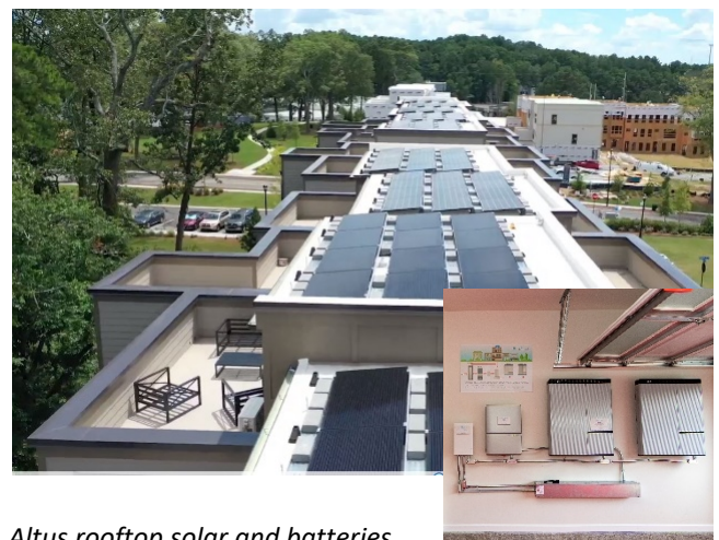
Altus rooftop solar and batteries. Images courtesy: Georgia Power .
