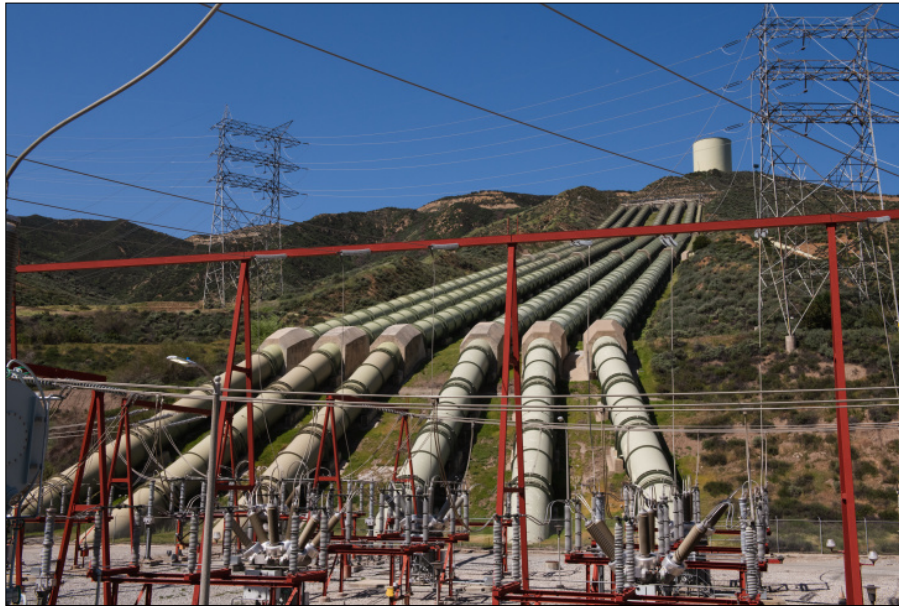
Figure 18: Pumped-storage plant of the Los Angeles Department of Water and Power in Castaic, California. 67
