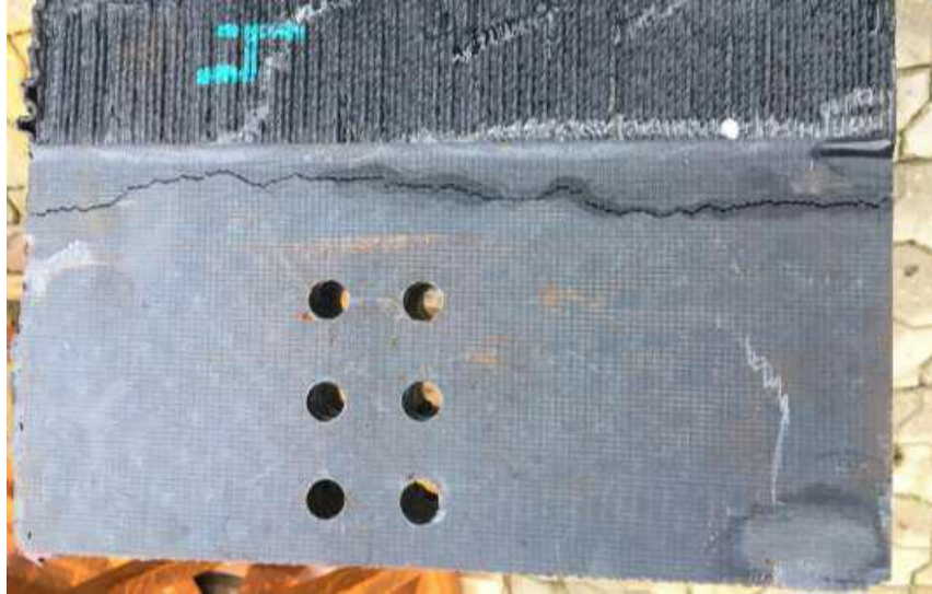
Figure 48. Composite V2 node failure Arm 4
