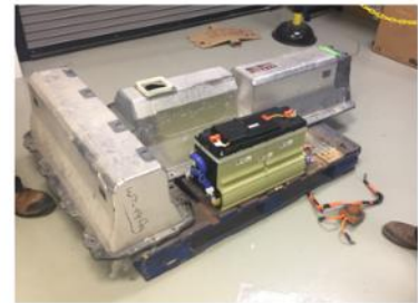
17) Cover Exposed Terminals
