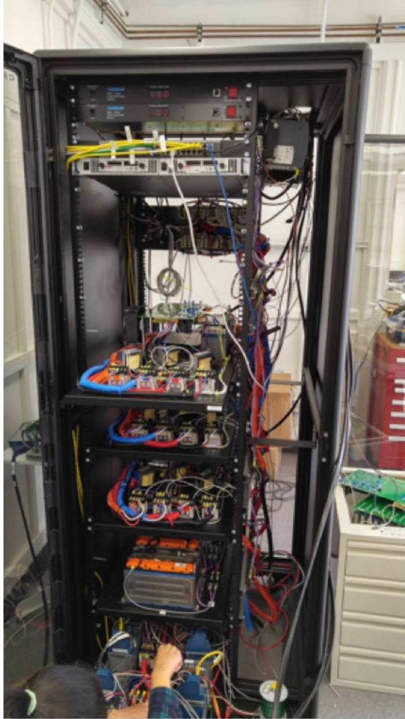
Figure 13. ORNL SI-GRID microgrid power systems test platform.
