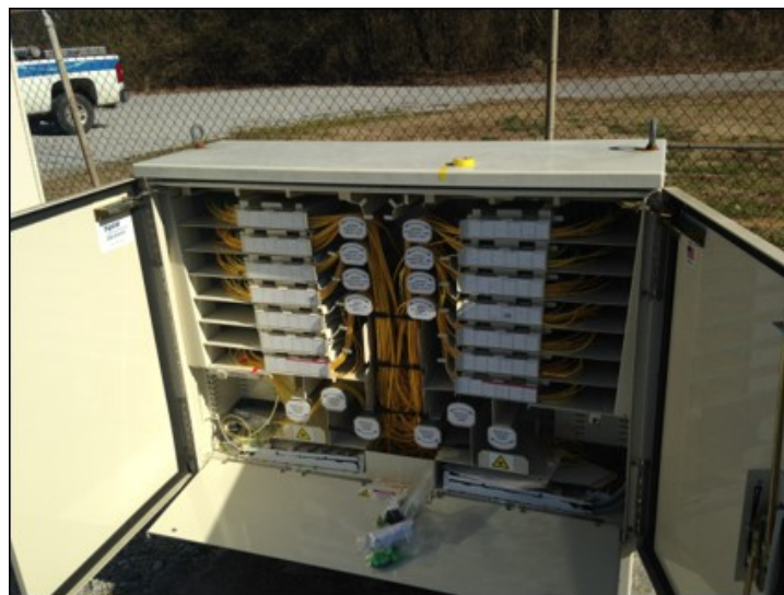
Figure 20. Loopbacks placed in single-mode fiber trays.
