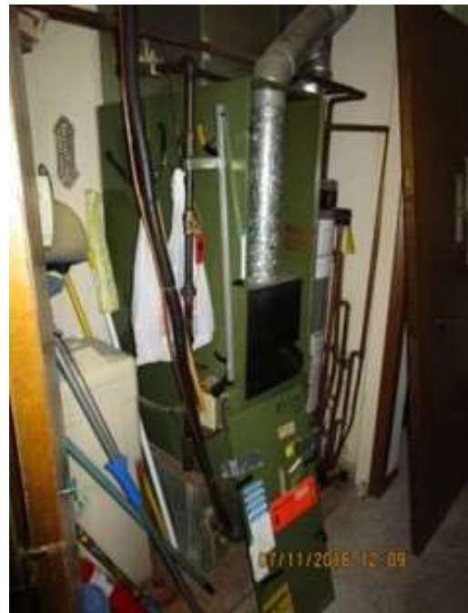
Figure 5.15. House MN2 furnace closet.
