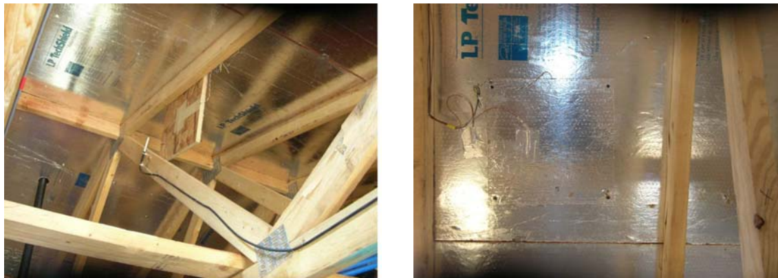
Figure 2. LP Techshield is the deck sheathing. A patch panel also made of Techshield [0.731-in (0.01857-m) thick] holds a heat flux transducer against the LP deck.
