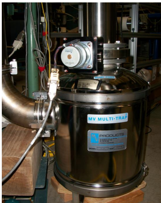
Fig. 11 Commercial filter-trap installed on the MAP vacuum line.
