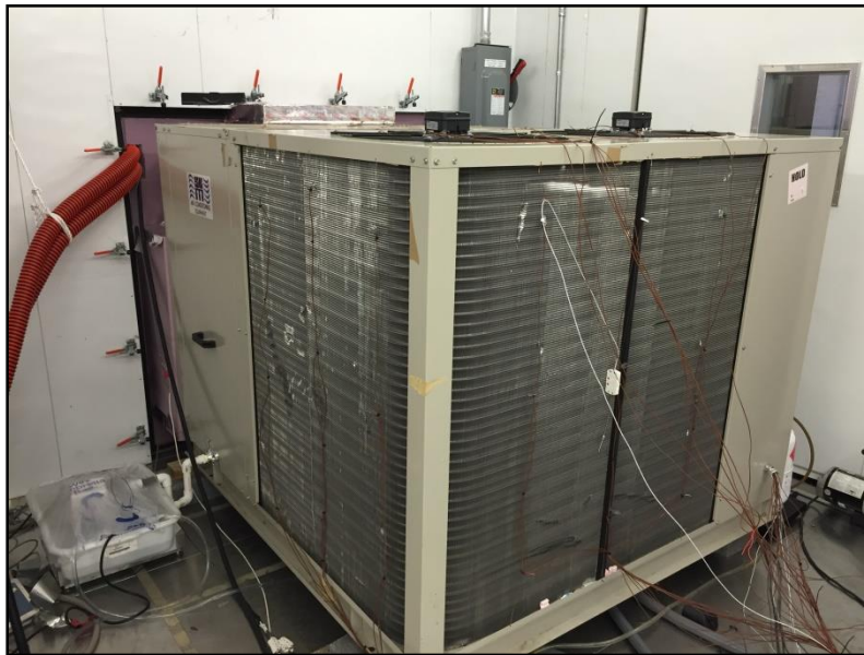
Figure C.1. As installed R-22 indoor unit.
