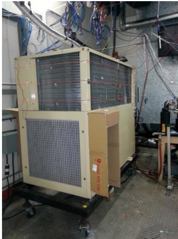
Figure 20 Pre-commercial heat pump prototype.
