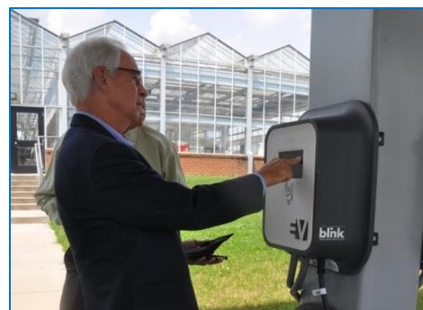
Figure 7: The University of Tennessee tour consisted of Living Light House, the Agriculture Campus' E-Bike Program, and the Agriculture Campus' solar-assisted EV charging stations.
