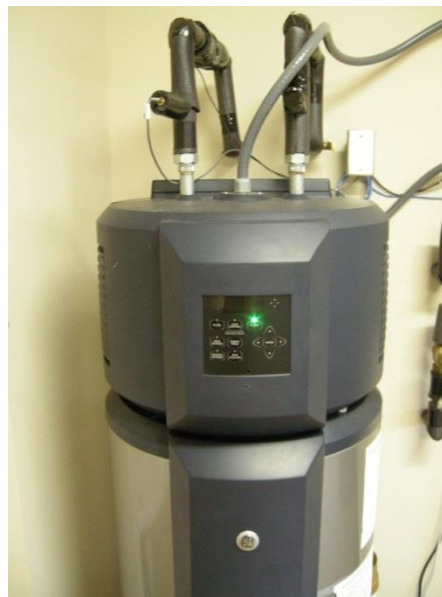
Fig. 1. GE Geospring HPWH at CC2.
