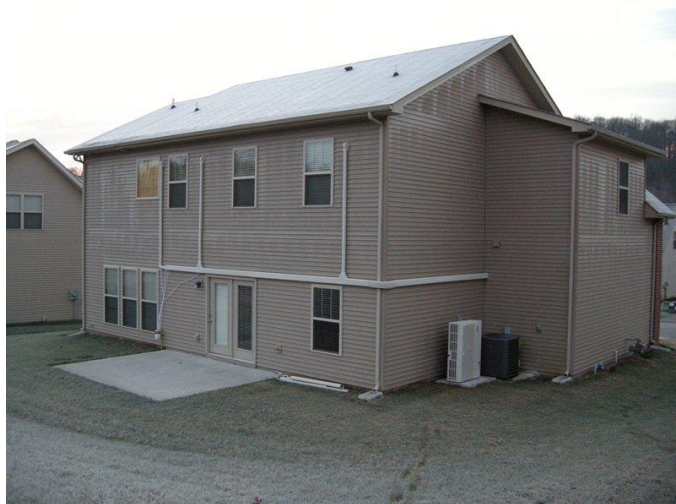
Fig. 2. Mitsubishi multi-split HVAC lines and compressor at CC2.
