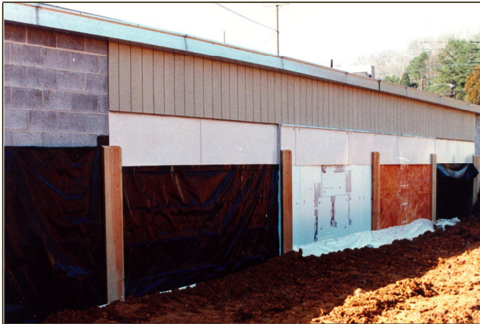
Fig. 2. Envelope Systems Research Apparatus at ORNL during construction in 1991.
